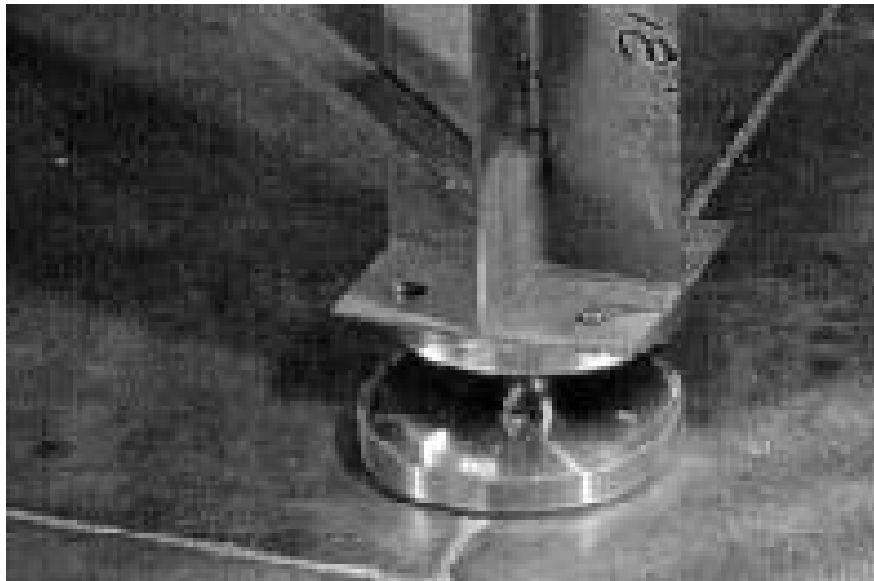
Figure 8. Close-up of Base Isolator
