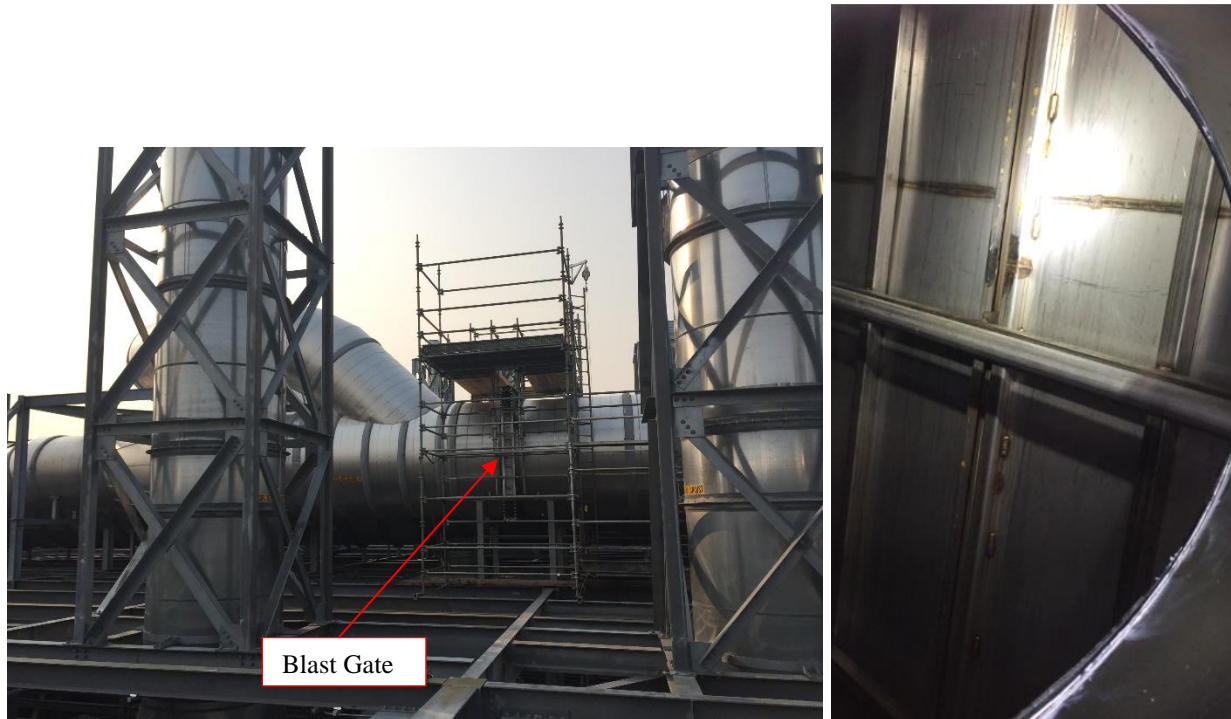
Figure 8: Overview of scaffold around blast gate (left); internal view of blast gate in support frame (right).
