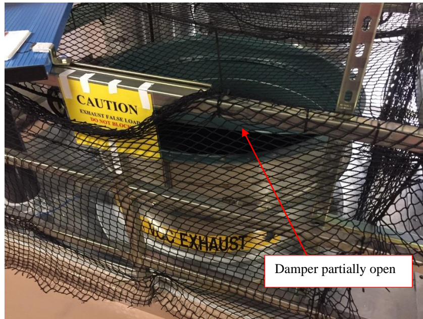
Figure 4: Photo of penetration, as seen on the subfab level. The EXVO duct terminates at this point with a partially opened damper.
